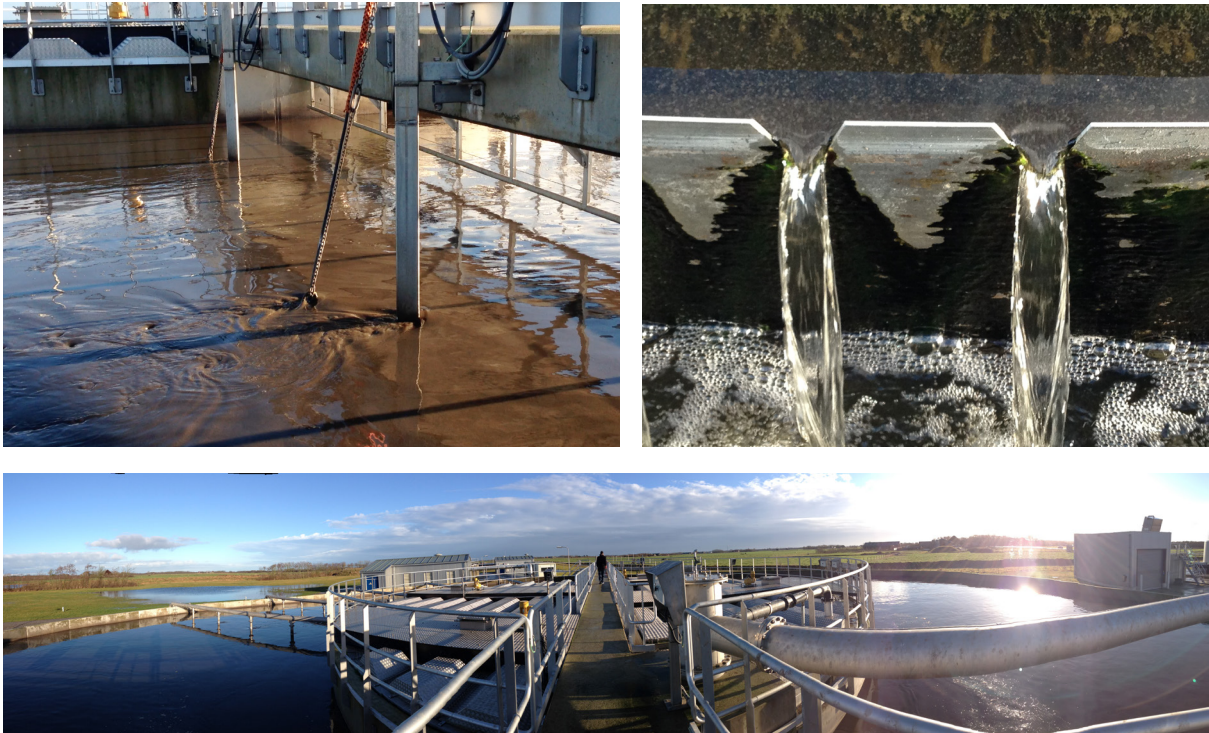
Figure 5.1: Pictures from our visit to HHNK facilities
