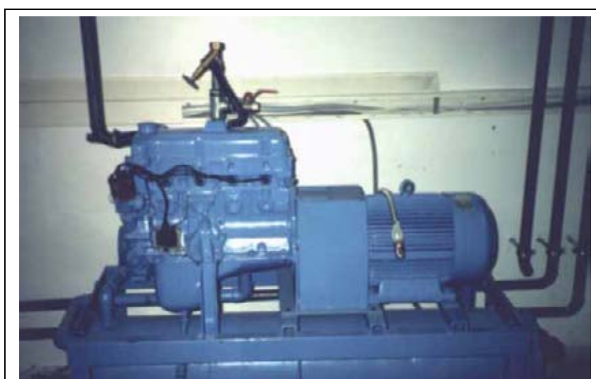
Figure 47: Co-generation unit (electricity and heat utilisation)
