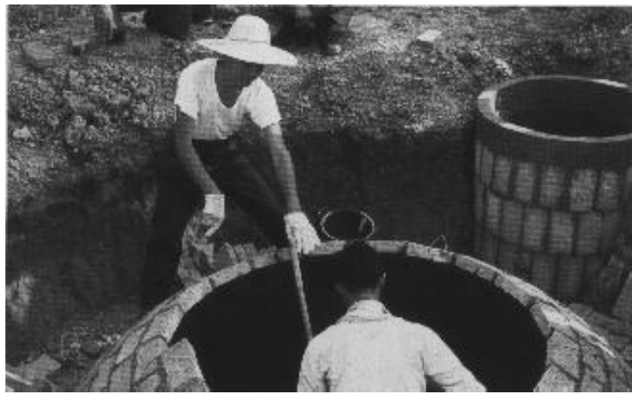
Figure 6: Installation of a Shanghai fixed-dome system near Shanghai, PR China Photo: L. Sasse
