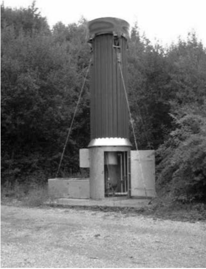
Figure 2.2 Gas flare for high temperature (1050°C) with hidden flame.
