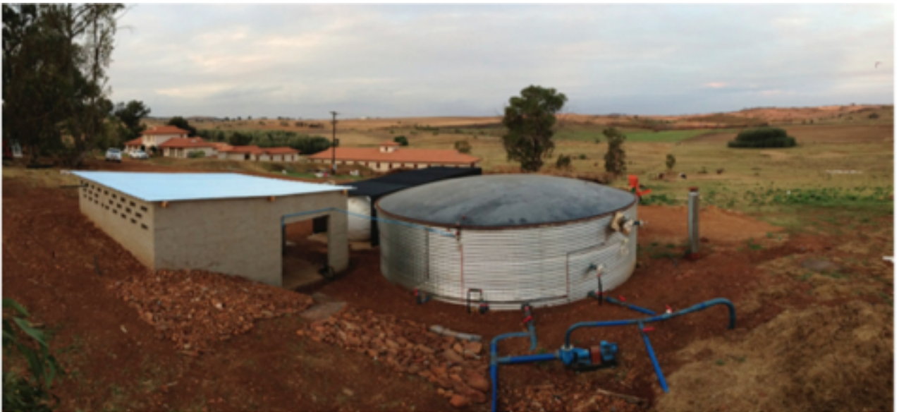
Figure 1: 150 kWh plant at Caesarsvlei
